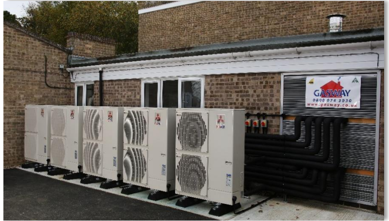
Example of a retired living scheme in East Suffolk that was fitted with a commercial air source heating system to improve the energy efficiency of the building.
